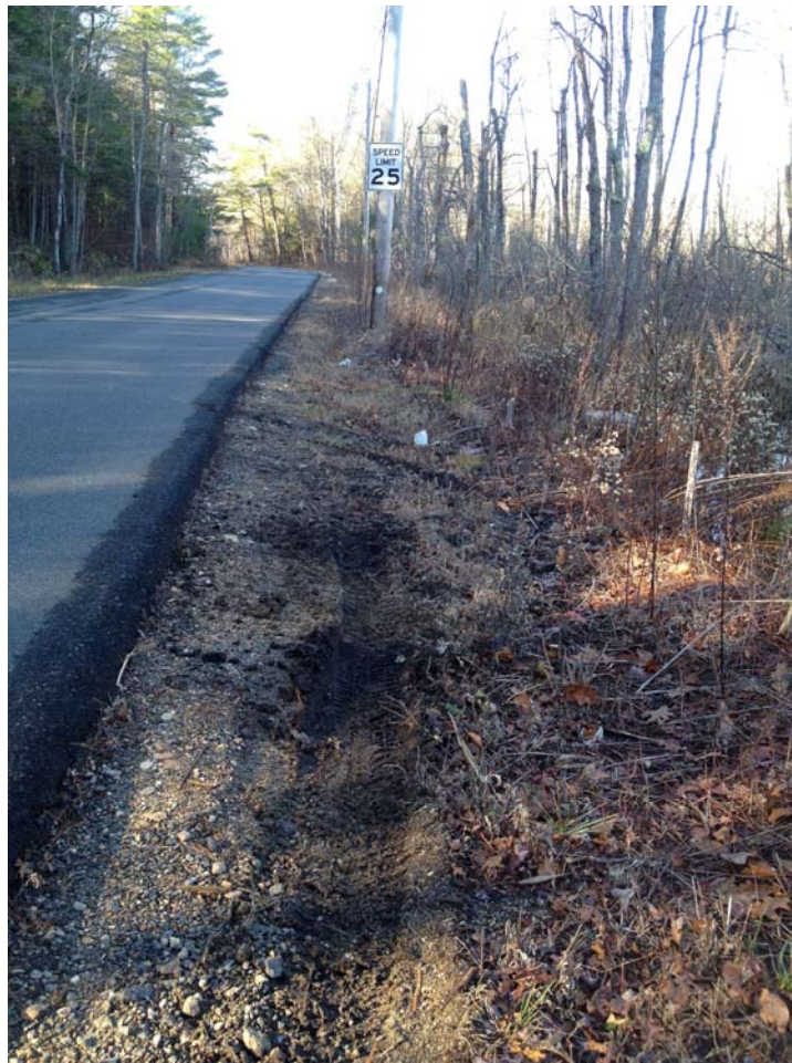
Road shoulder on north side of Pine Street in study area. Erosion control sock and stakes remain in place but have deteriorated
